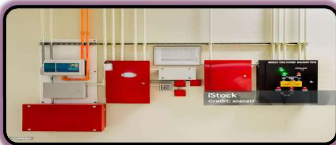
Fire Aspirating System
